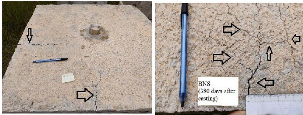
Fig. 7. Images of the BNS sample with surface cracks after one year of exposure in the natural environment.
